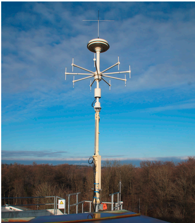
Combined R&S®ADD157, R&S®ADD050SR and R&S®ADD070 direction finding antennas, installed in Grünwald near Munich, Germany.
