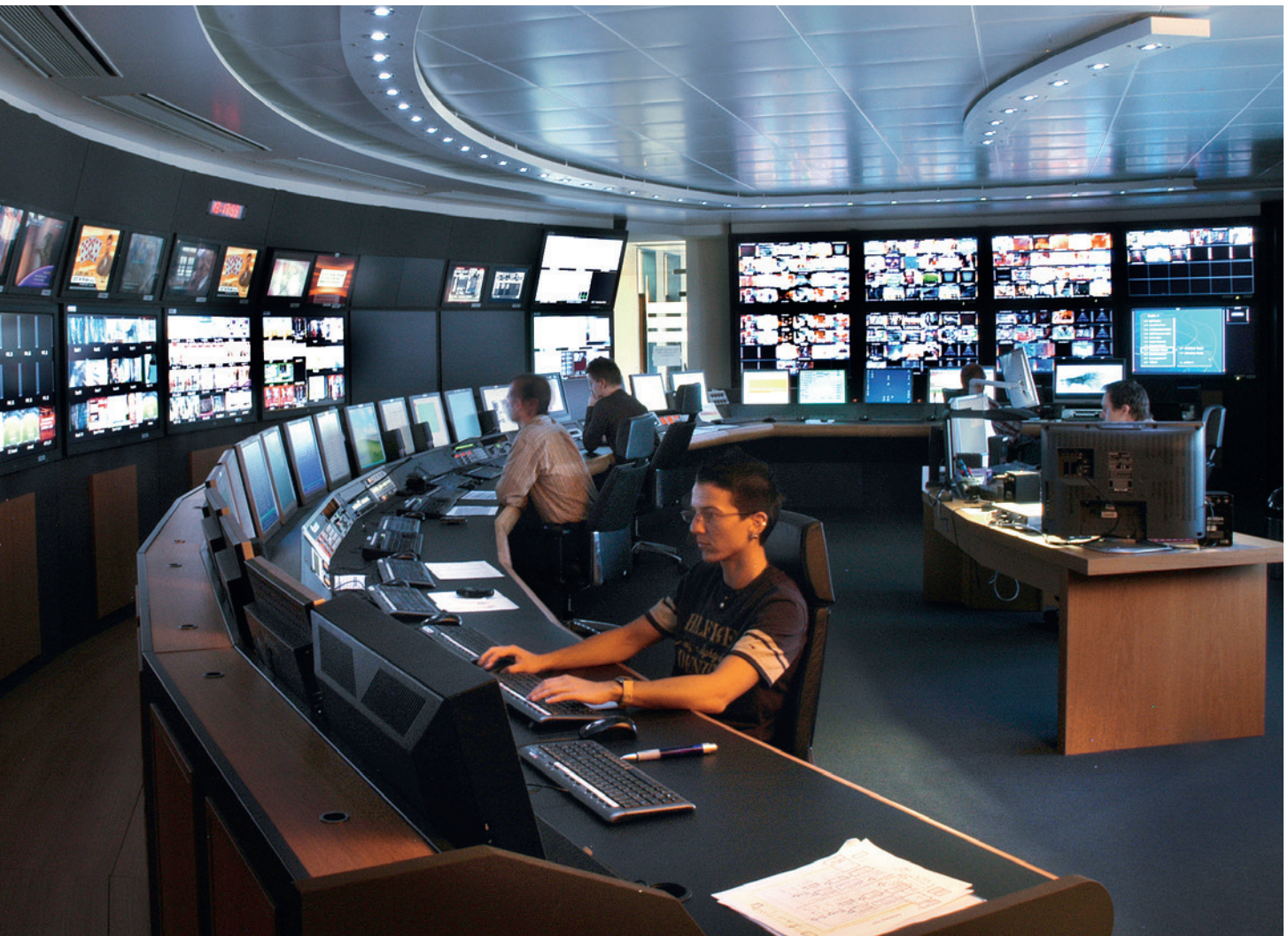
Master control room (MCR)
