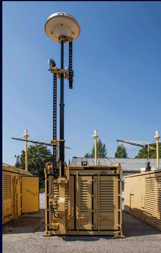
R&S®ESMW installed in a COMINT shelter
